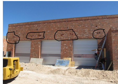
Installation bolts for overhead door
